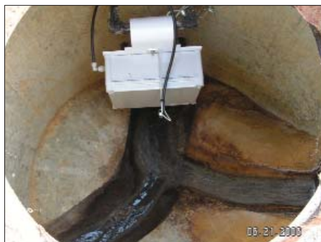
G2 PANEL (INSTALLED IN GROUND)
