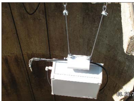
G2 PANEL (INSTALLED IN PUMP STATION)
